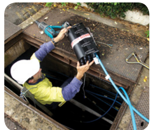
Use of existing pit in Brunswick, Victoria, one of the First Release Sites.
