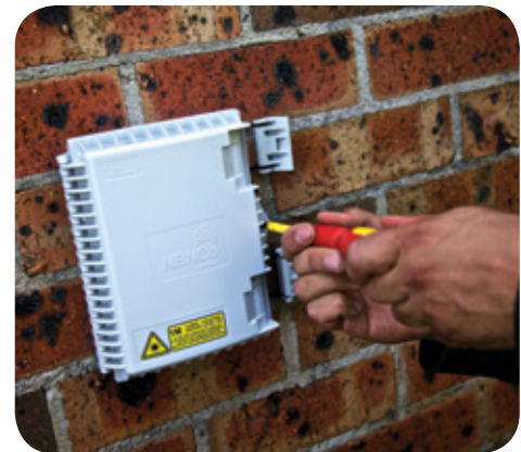
A typical Premises Connection Device, Kiama, New South Wales, one of the First Release Sites.
